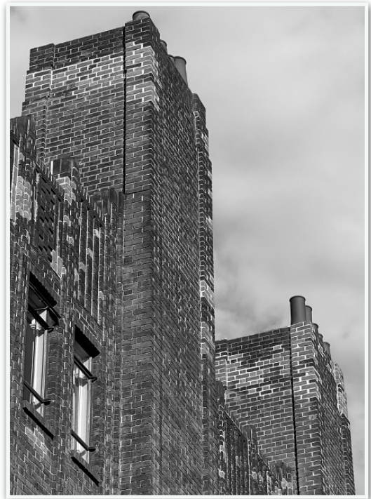
Although in black and white, the crude pointing is clear.
